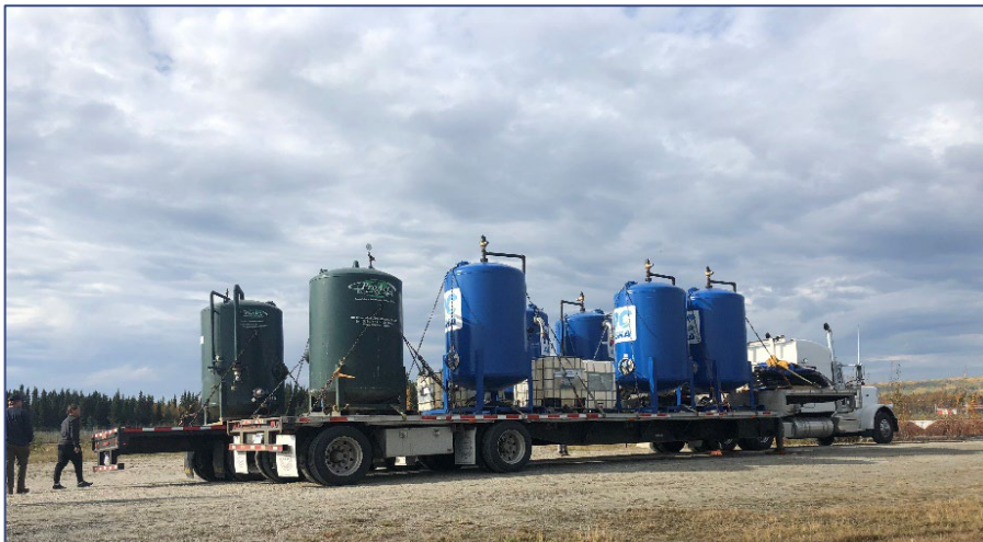
Exhibit 2-3: Onsite water treatment system (September 9, 2019)
